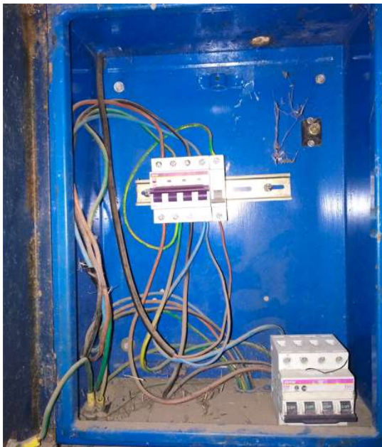
Fig. 73. Interior tablero principal
