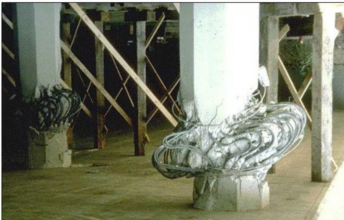
Figura 2.53 - Zona de empalme colapsada [Álvarez J.C., S.F. Breña (2017)]
